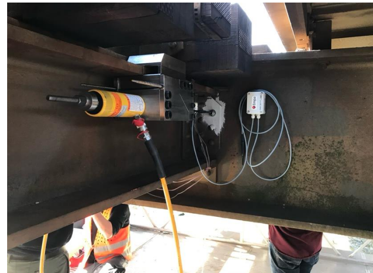
Aabach rail bridge, fatigue reinforcement of stringer-crossbeam connections with prestressed CFRP rods
