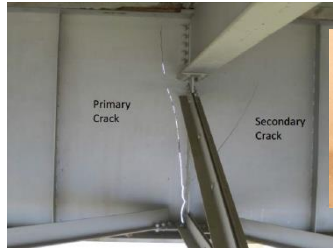
Fatigue cracks in the Diefenbaker Bridge
